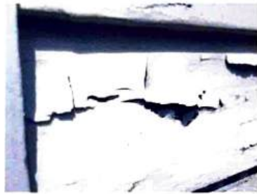
Lead paint coming as flakes
