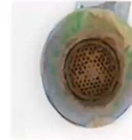
scaling on pipe & fittings?
