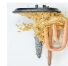
scaling on geyser heat coil
