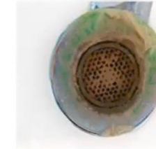
scaling on pipe & fittings?
